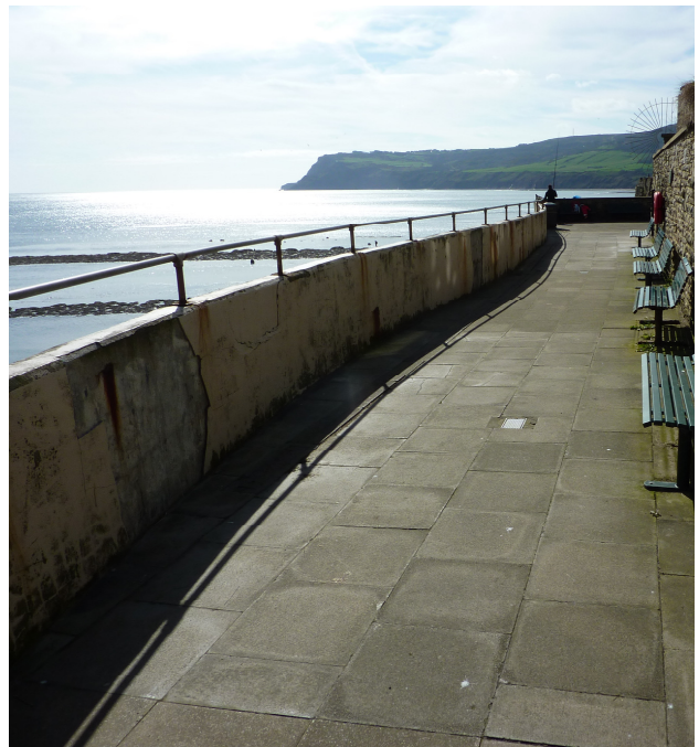
View south along rear of parapet wall showing cracks, rust staining and loss of surface.
