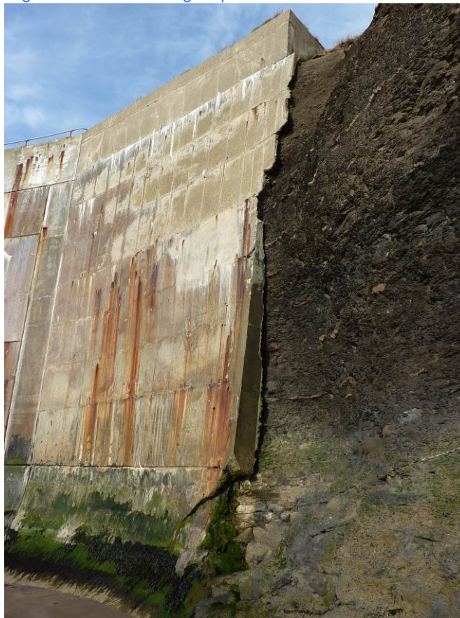
View South of the interface between the cliff and the sea walls showing erosion of the cliff leading to outflanking of the sea wall and damage to the edge of the wall. The edge repair is visible on the lower half of the wall.
