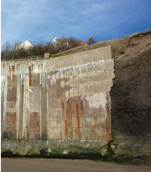
View of intersection between cliff and sea wall showing rust and white staining
